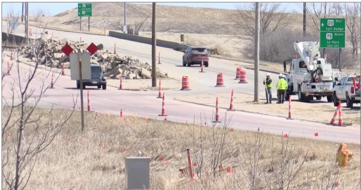
Traffic rerouting due to construction on Highway 20 in Sioux City. Photo credit: Siouxland Proud, 11/21/2023.
